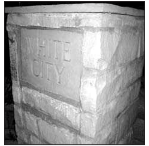
After months of trying to find a mason to repair this monument, White City Chair Troy Blundell did the work himself.
